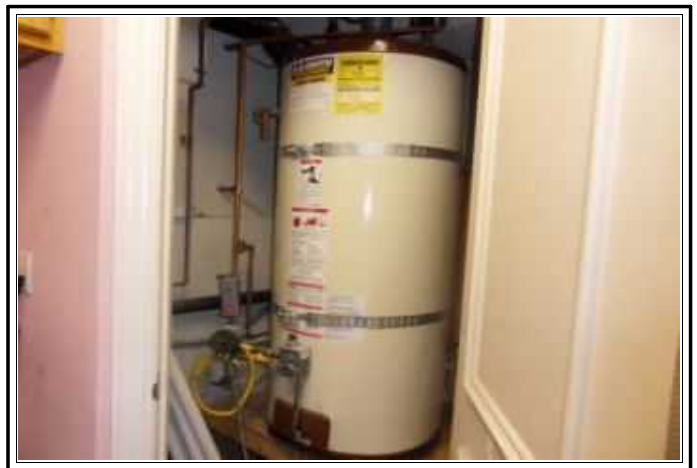
Water heater, double strapped
